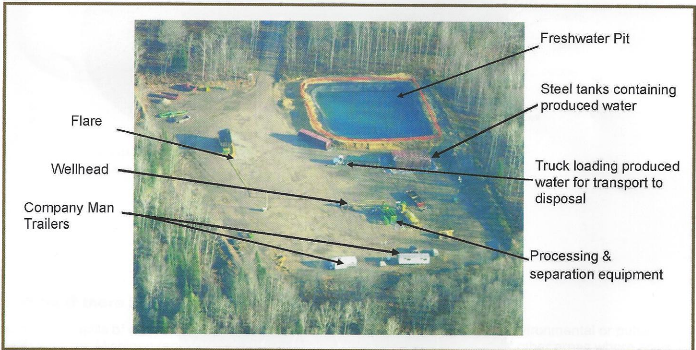
Aerial photograph of a Utica- Collingwood well during "flowback" after hydraulic fracturing is complete. The Freshwater pit, shown in the upper right, remains in place from the hydraulic fracturing but is not used during the flowback stage.
